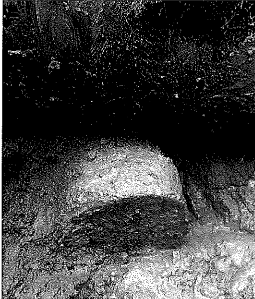
Figure 9: Piece of rock that causes a dent in the pipeline.
